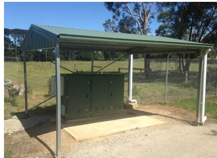
Chlorinator cabinet under the shade
