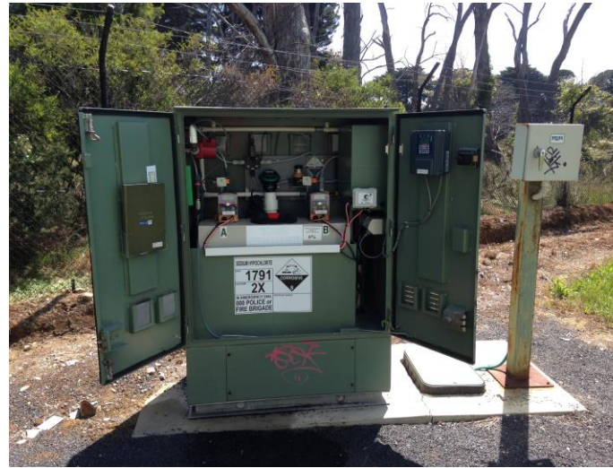
Chlorinator cabinet with s. hypo storage under the cabinet
